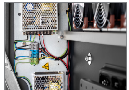
Cabling according to VDE guidelines
